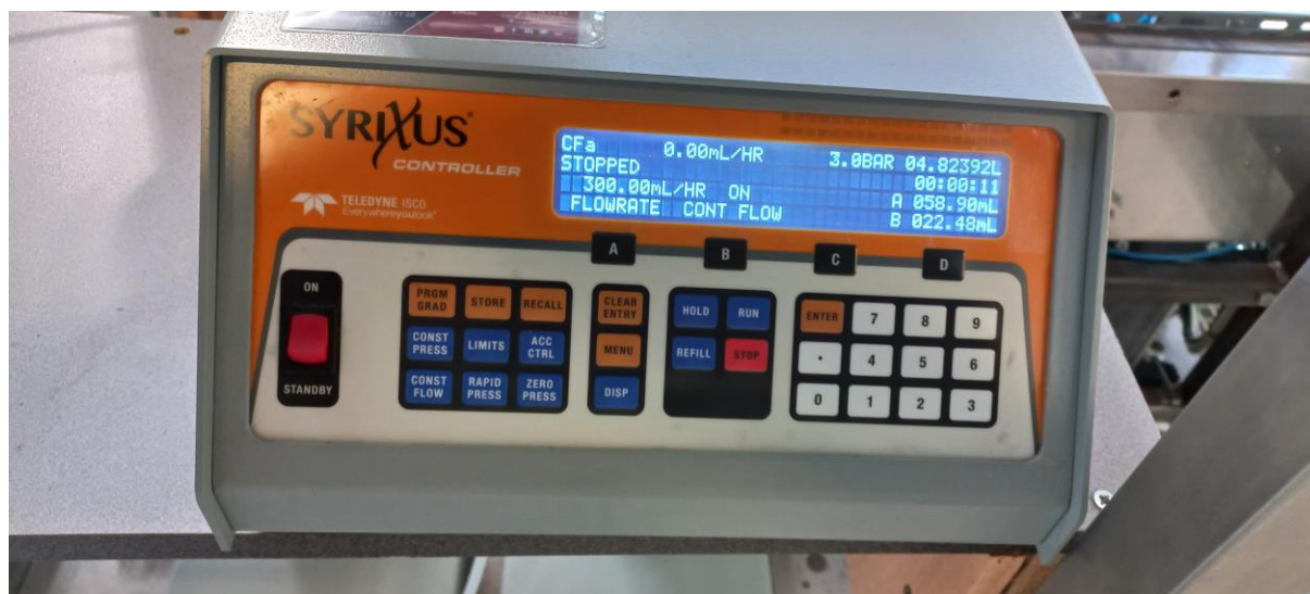
Figure 4: Main control panel of the pumping system
