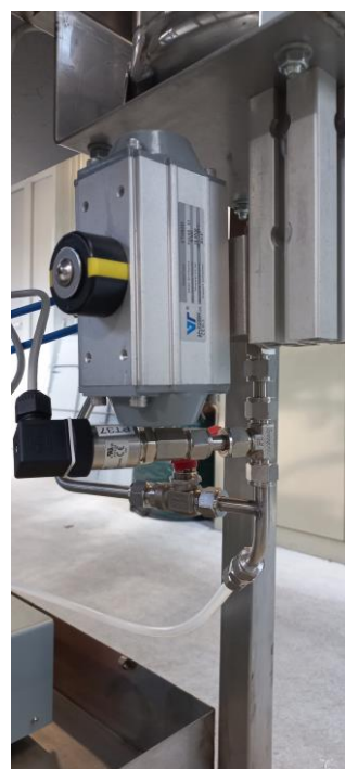
Figure 3: Solenoid valve for tank selection
