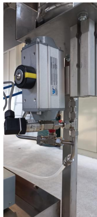
Figure 3: Solenoid valve for tank selection
