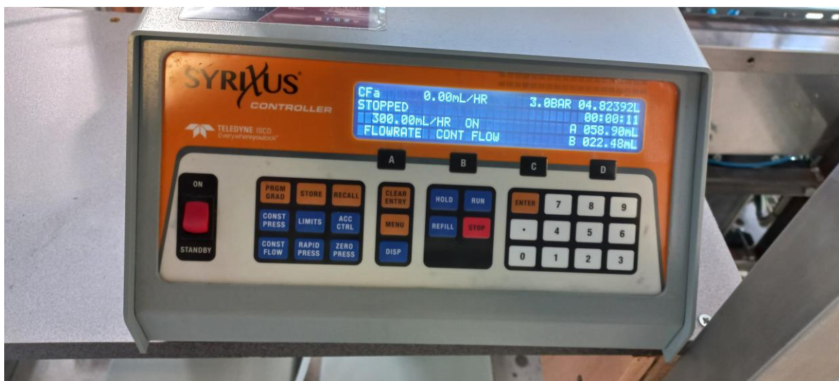
Figure 4: Main control panel of the pumping system
