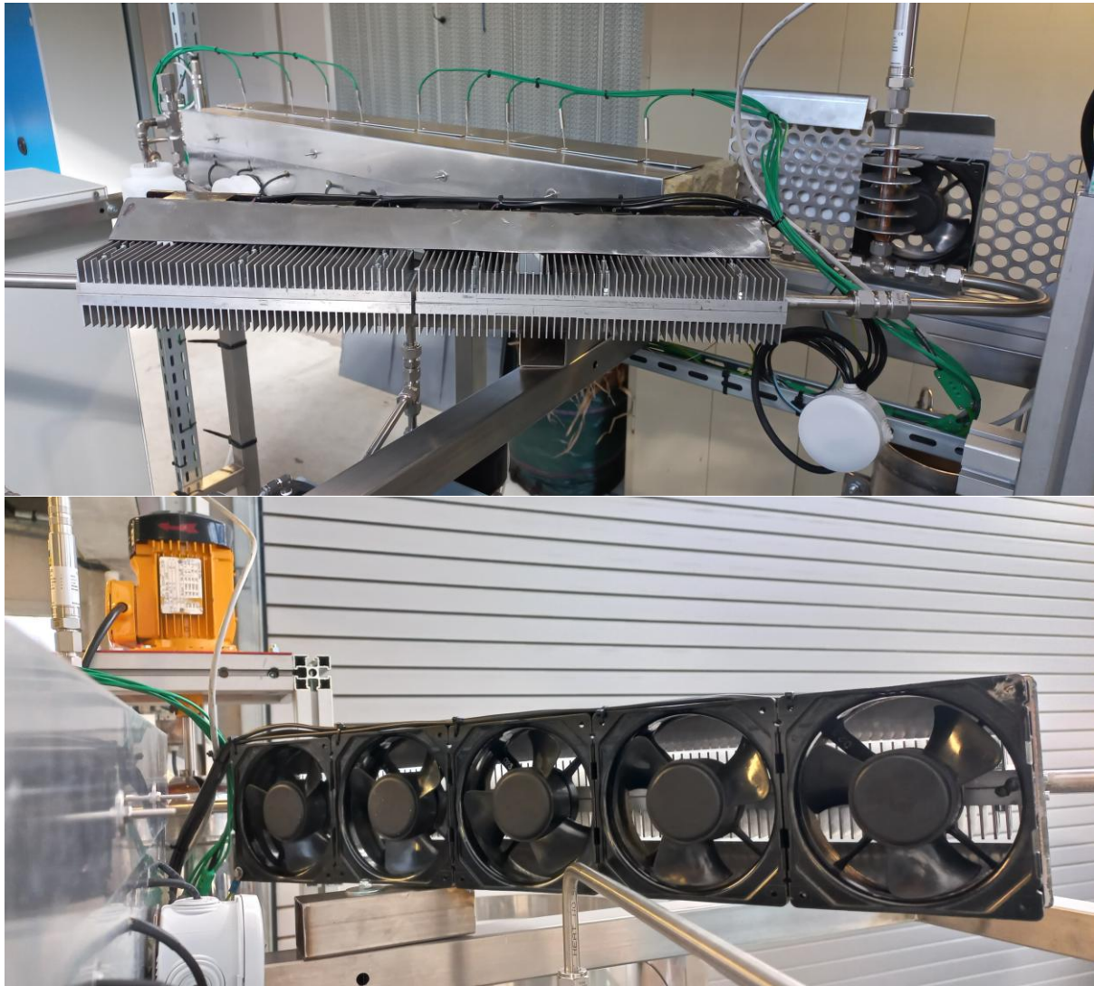
Figure 11: Front and back view of the cooling system mounted on the continuous unit's frame
